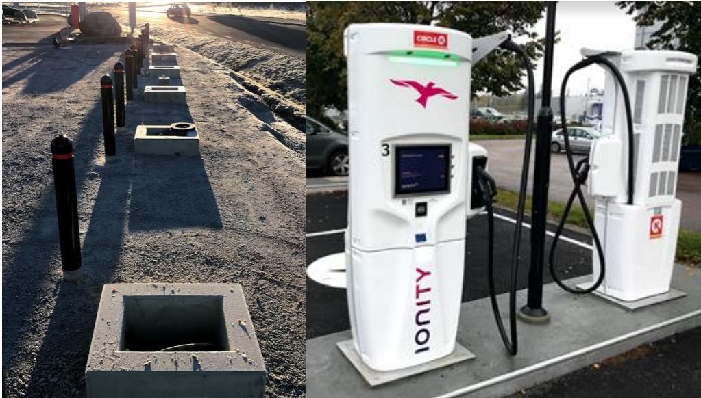
Different stages of installation. Rightmost picture showing a Tritium charger installed using an adaptor between the foundation top and base of charging station.
