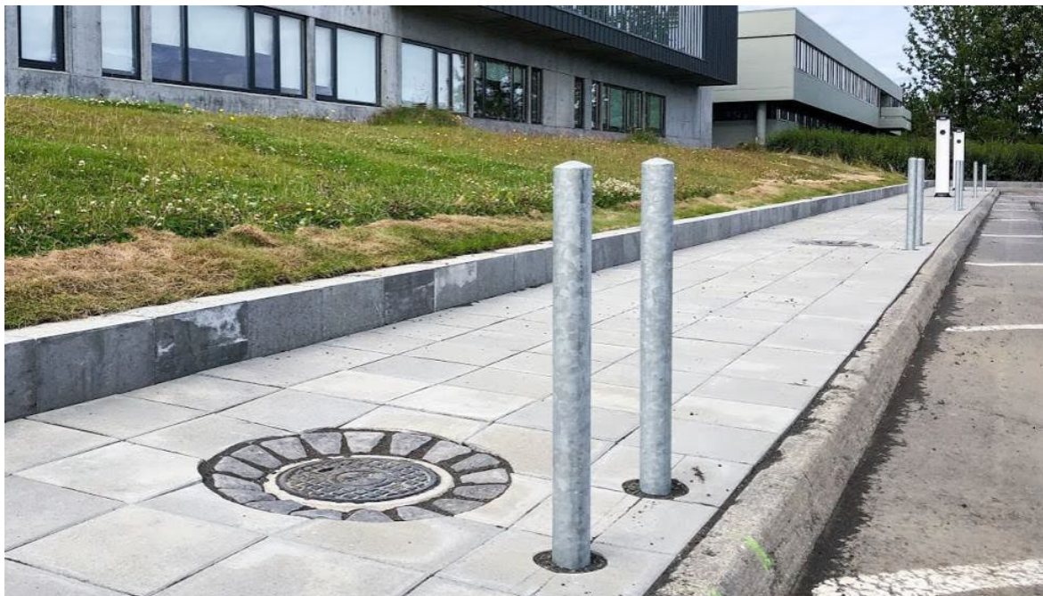
A charging ready street in Reykjavik, Iceland showing 3 future proof, scalable, pre-prepared Unimi-1bases with crash protections. In the distance, two installed EV charging stations serving current EV charging demand
